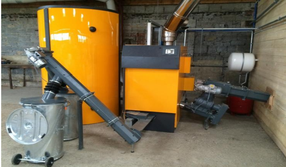
Figure II-3: Chaudière à biomasse
