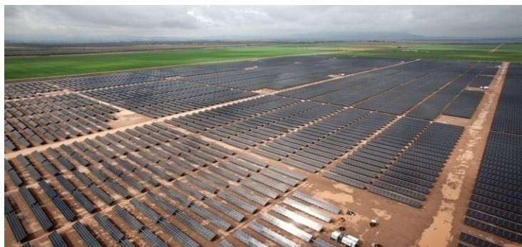
Figure I.10 Un champ photovoltaïque
